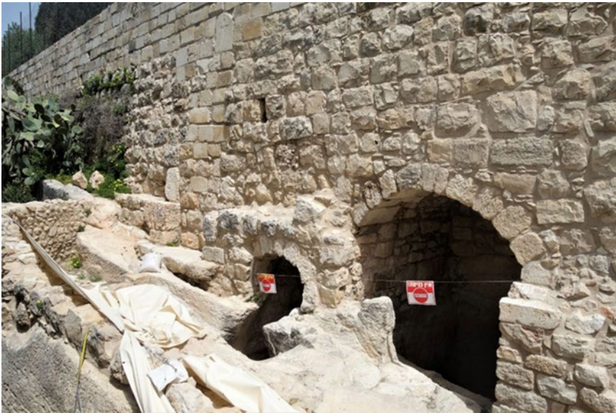
Fig 2.7: The recently restored double miqveh , with sealed postern to the left, on a ledge, at the base of the modern wall, 3m above the level of the Protestant cemetery.
